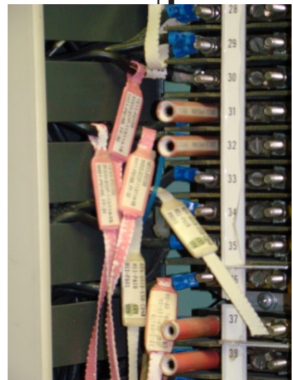
Figure 5: Painted terminal jacks with paper labels.
